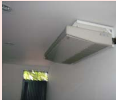
Air conditioning unit inside the computer lab
