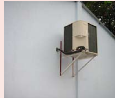
Our Rotary grant enabled the school to install this new air conditioning unit
